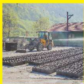
FACTORY OF CONCRETE PRODUCTS
